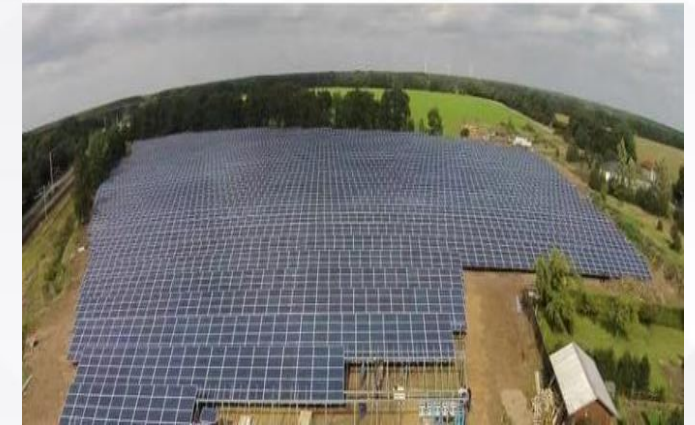
36MW 2022 in Germany
