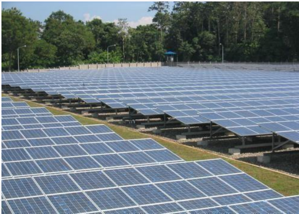
14.5MW 2011 in Italy
